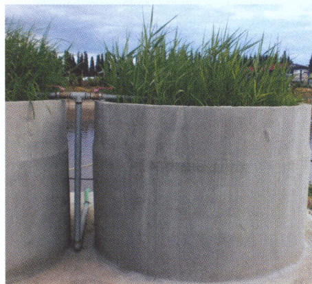
Vertical flow reed beds provide direct treatment of the organic load in the lagoon. Each bed is 6.5-feet in diameter and 5-feet high, and planted with Phragmites Australis spp.
